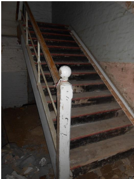
Figure 2 - original decor and staircase from MOD use
